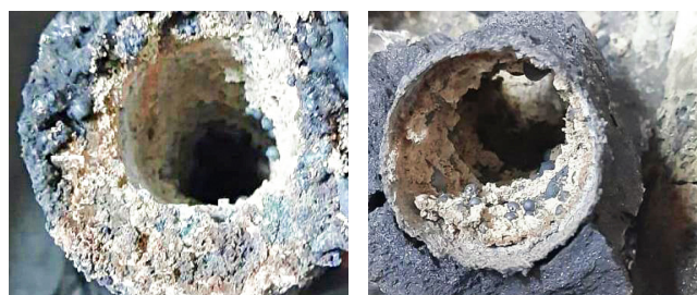
Typical Clogging Occurred
